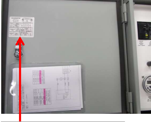
Inside door of the control panel. Silver label, black print.
